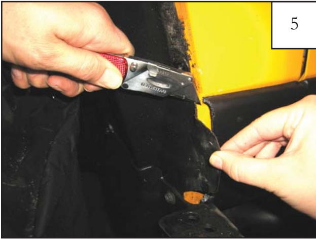
Using a utility knife, cut splash guard flush with edge of a sheet metal.
